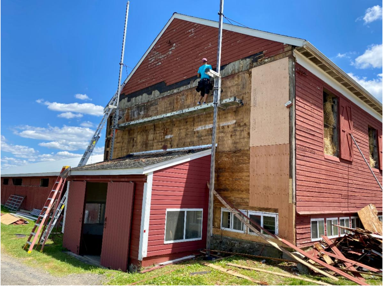
Old siding was removed and new siding was installed at the Town Line Farm Preserve
